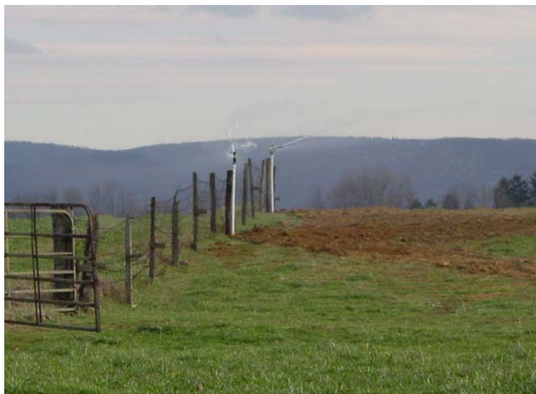
Sprinkler system installed at the farm of Charles Carothers III to handle barnyard runoff.
